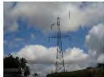
818 Power Cable Line
