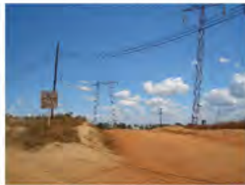
836 Power Line Cable
