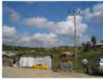
820 Power Cable Line
