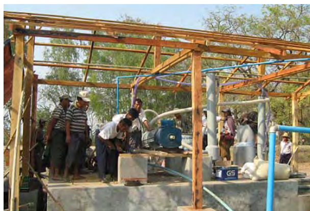
Construction of the husk biogas power generation now under way. The project constructed the main part only while ancillaries were done by the villagers.
