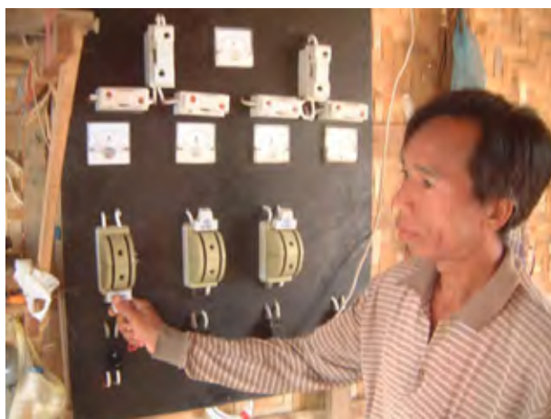
Generator-operator can cause damage at the place where there is an unauthorized use of electricity by changing from AC to DC when there occurs fluctuation of voltage.
