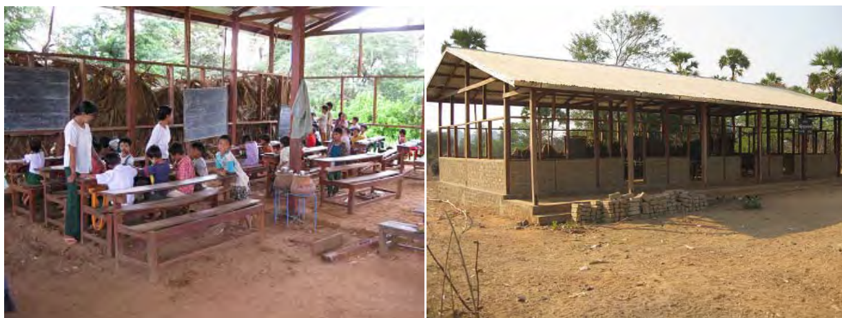
Photo in the left shows the school building with temporary wall wherein the pupils already started studying. Then the villagers contributed a lot, one of the contribution is the wall. They have donated sand stone slabs which have been used as wall materials (see the right photo). The work still continues as of January 2010.
