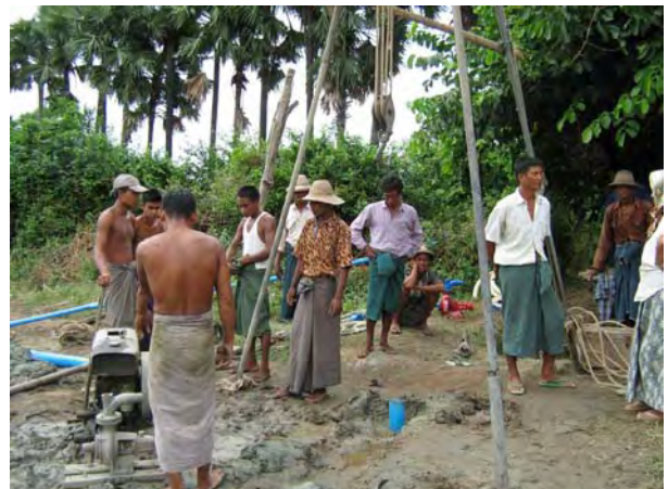
Tubewell Drilling (Magyi Village): A construction of well is being done by using traditional method. The water is to be used for vegetable irrigation.
