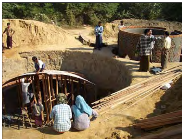
Construction of the Main Tank (forefront) wherein bio-gas production by cow dung is to be made, and disposal tank (right above) where fermented cow dung is to be discharged. The villagers contributed in the excavation work.
