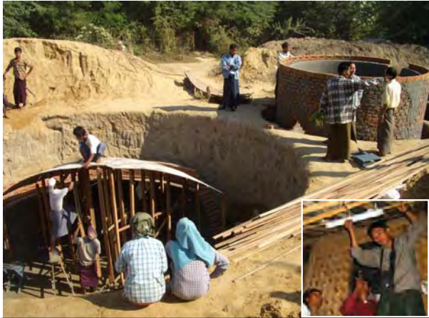
Bio-gas Plant Construction (Khaungkawe Village): They are constructing the first tank wherein cow dung is to produce bio gas to run diesel engine for power generation.
