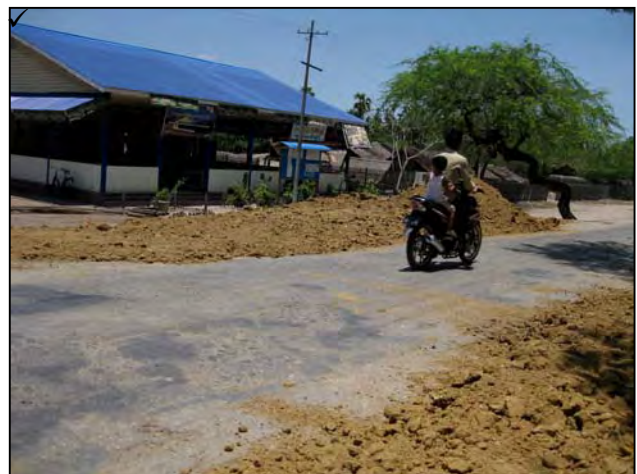
Photo (2) - Scene of road extension work being carried out by the committee after getting suggestions.
