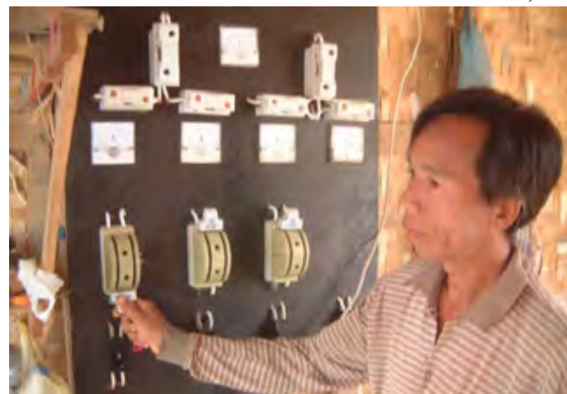
Photo 2: Generator-operator can cause damage at the place where there is an unauthorized use of electricity by changing from AC to DC when there occurs fluctuation of voltage.
