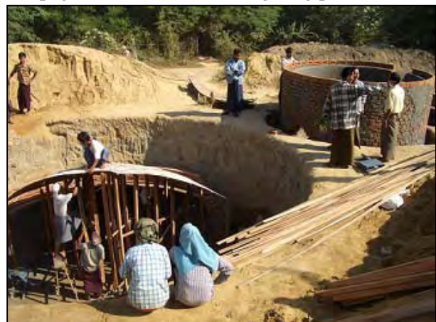
Photo 1: Construction of the Main Tank (forefront) wherein bio-gas production by cow dung is to be made, and disposal tank (right above) where fermented cow dung is to be discharged.
