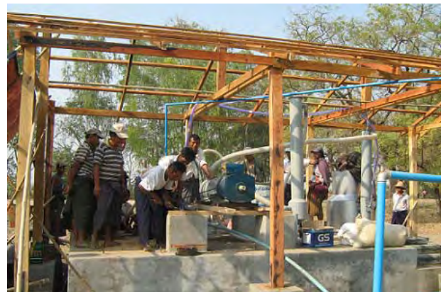
Photo 2: Construction of the husk biogas power generation now under way. The project constructed the main part only while ancillaries were done by the villagers.
