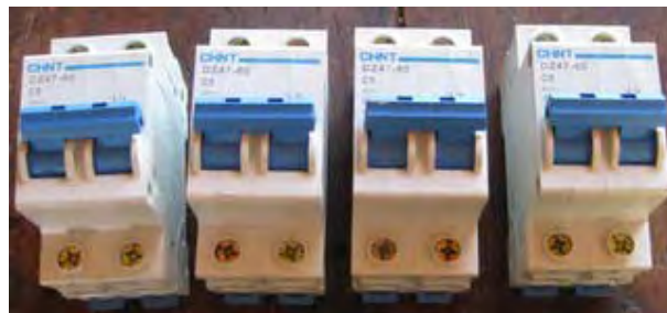
Photo 1: Instead of big breakers, such small breakers were installed to protect the generator from overloading.
