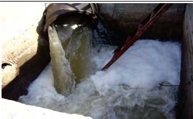
15. Discharge tank of Shurafah reuse pump station
