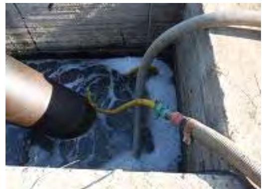
MBD Operation in Suction Chamber
