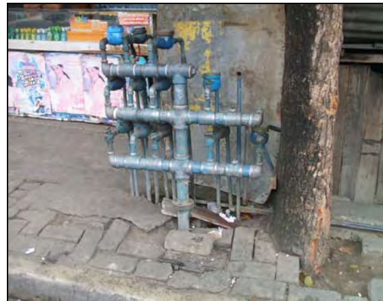
Figure II-24 Conditions of Stub-out
