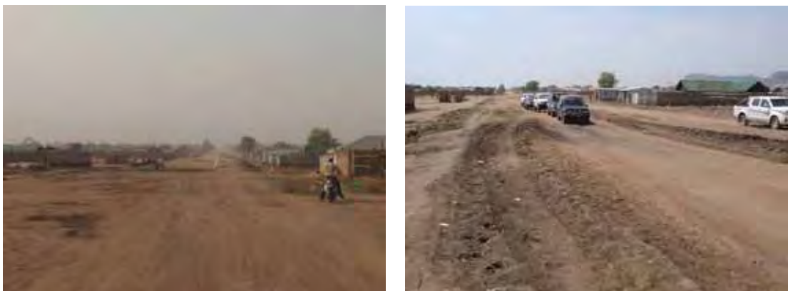
Photo 25.2.2-2 Road Condition in Munuki Extension Road
