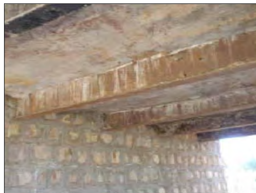
Steel H-Beam with Corroded Section/Section Loss (No.10)
