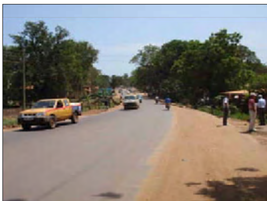
Road Narrows at Culvert Section of Paved Road (No. 9)
