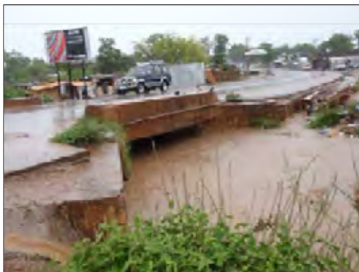
Insufficient Freeboard on Culverts During Rain (No.17)
