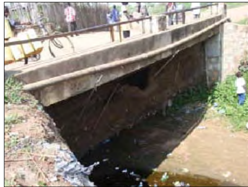
1-Span 2-Lane RC Slab on Steel H-Beam Bridge with Masonry Abutments (No.7)
