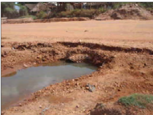
Embankment Erosion at Temporary Steel Pipe Culvert Narrows Road (No. 14)
