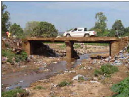
2-Span 1-Lane RC Slab on Steel H-Beam Bridge with Masonry Abutments and Pier (No.6)
