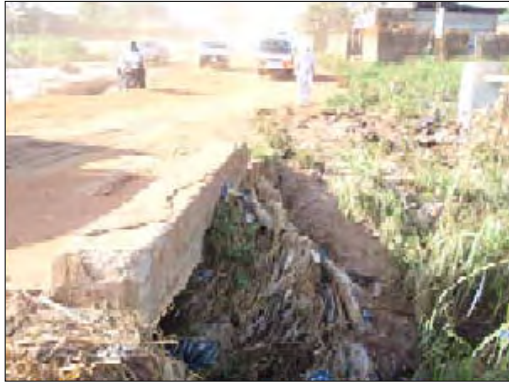
Debris/Garbage Blocking the Upstream Opening (No.12)
