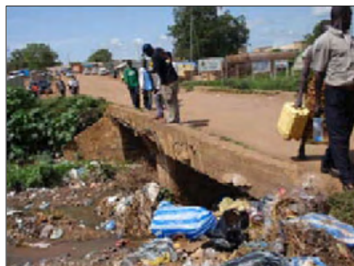
Debris/Garbage Accumulating at Upstream Side (No.6)
