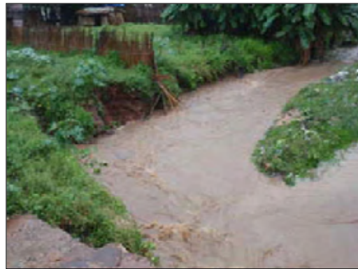
Scouring of Upstream Bank During Rain (No.9)
