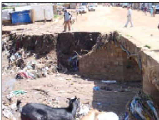
Scouring of Road and Abutment at Upstream Side (No.6)
