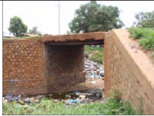
1-Span 1-Lane RC Slab on Steel H-Beam Bridge with Masonry Abutments (No.2)
