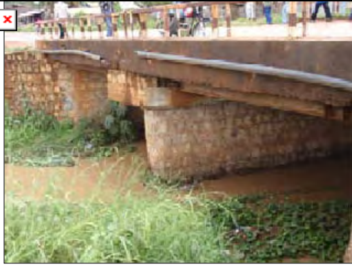
2-Span 2-Lane RC Slab on Steel H-Beam Bridge with Masonry Abutments and Pier (No.1)
