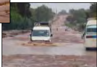
Culvert No. 14 – Flooded during heavy rain
