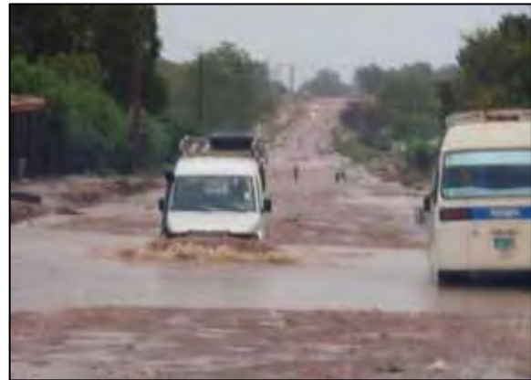
Typical Road Condition During Rain
