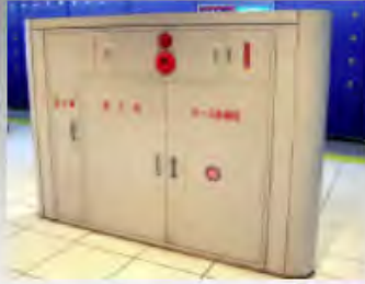
Inner Hydrant in Station
