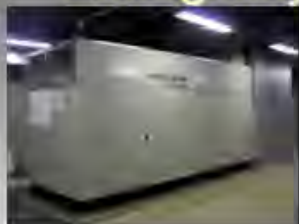
Emergency Power Generator
