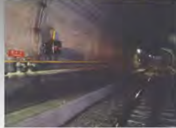
Siamese Connection in Tunnel
