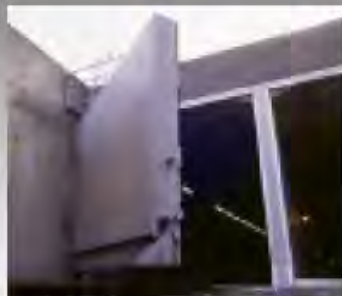
Water Stop Iron Door at the Entrance of Tunnel
