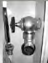
Siamese Connection in Station (50m)
