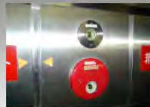
Push Button Alarm
