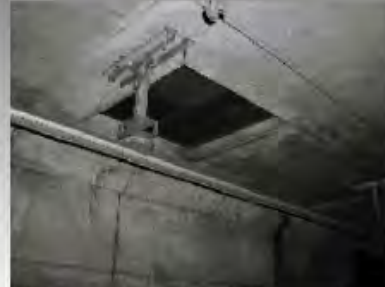
Exhaust Duct in Tunnel Source: Sendai City Transport Bureau, Japan
