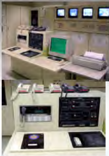
Monitor, Telephone and Public Address
