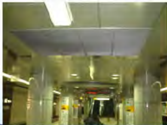
Duct in Platform Source: Tokyo Metropolitan Gov. Bureau of Transportation
