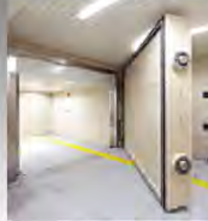
Water Stop Flap Door at the Passage Way
