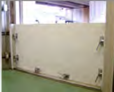
Water Stop Panel at the Entrance of Station
