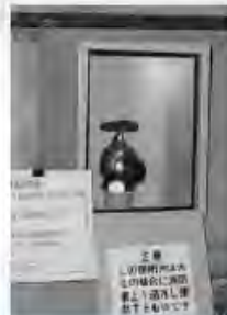
Siamese Connection in Tunnel (less than 500m) Example: Metro in Tokyo, 200m interval
