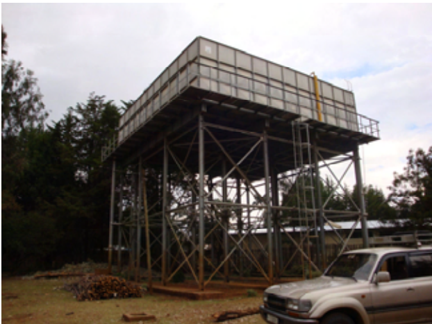
East Gojam No.6: Bichena 配水池
