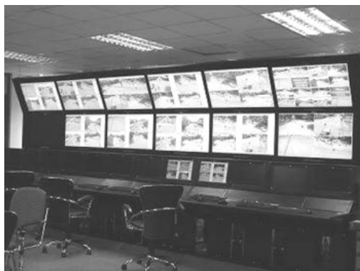
Figure 6.4.2 Traffic Monitoring Centre
