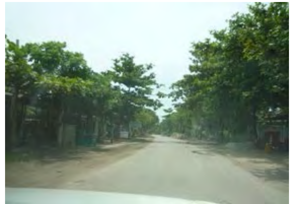
Photo-2 Condition of NH12B
