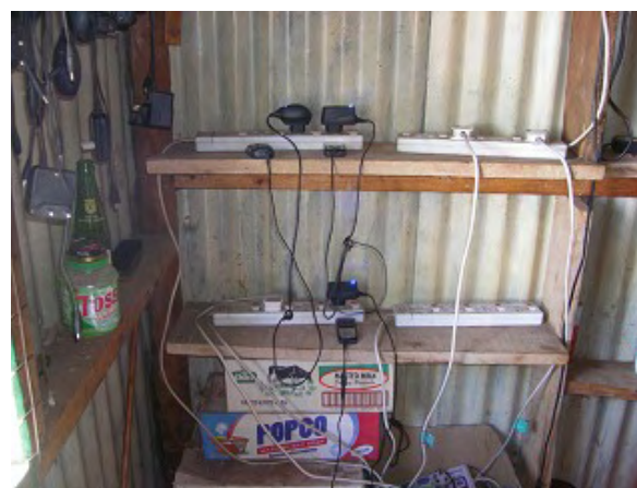
Battery charging service located near the dispensary
