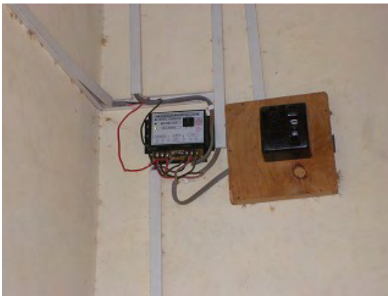
Photovoltaic generation controller
