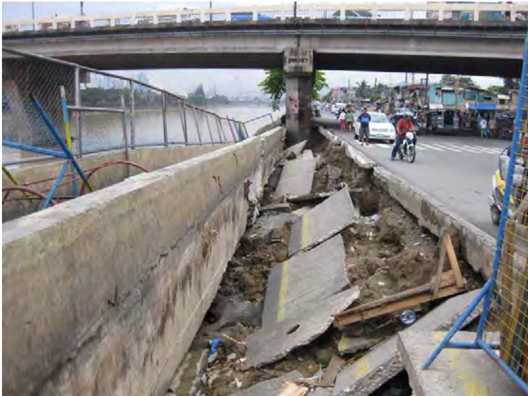
Photo-6 Damaged Structure during Ondoy due to Clogging of Road Drain Pipes at Left-side of Mangahan Floodway
