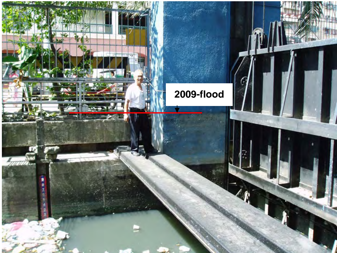
Photo-3 Flood Gate, Pandacan Pumping Station (Metro Manila)
