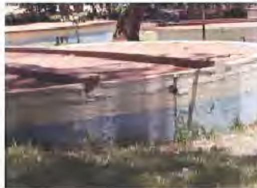
EWASCO water storage tanks in Embu
