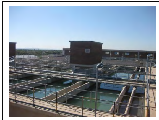
Mmamashia Water Treatment Works
