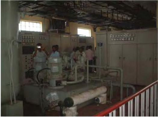
Fig. 10 Appearance of the Inside of the Power Plant
