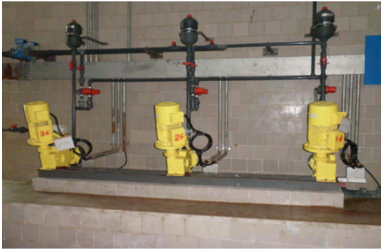
Chlorine dosage facility
