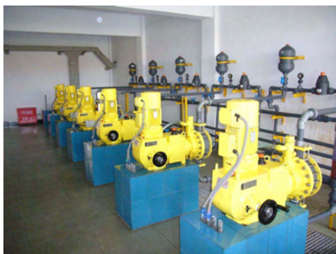
Chlorine dosage facility at Fengshouba Plant
