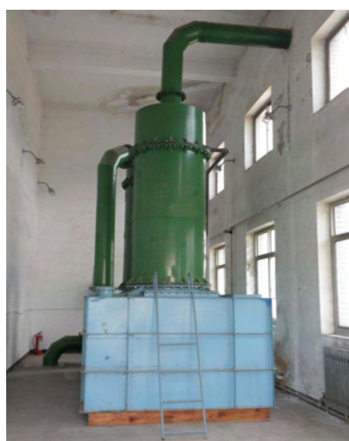
Chlorine dosage facility installed by the project in Qianxi County
