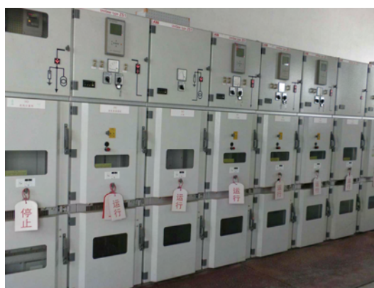
Power distribution panel installed by the project in Guye District
