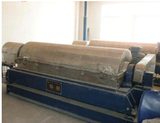
Processing facility for sludge
