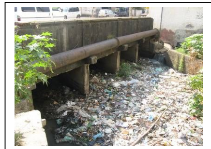
Drainages with garbage (Open drainage in Serpentine area)
