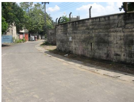
Open side drains with slab lids for easy operation and maintenance (Attidiya)
