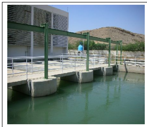
Manghopir Pumping Station
