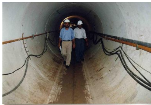
Underground drainage pipe at Unity Place
