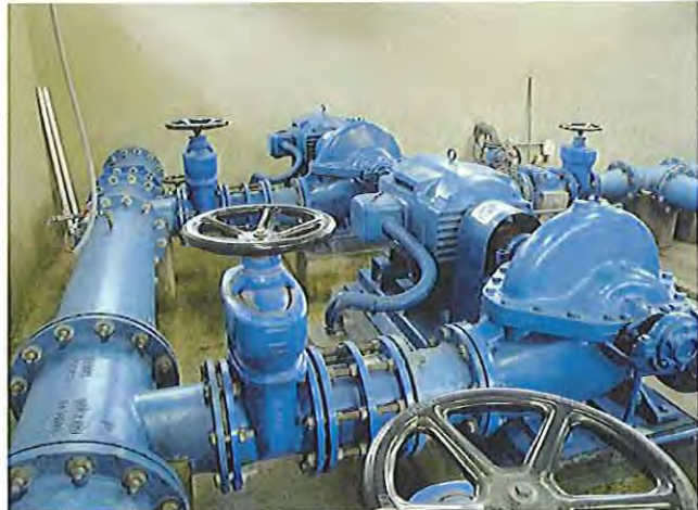
Water distribution pump (Rimac District, Lima)
