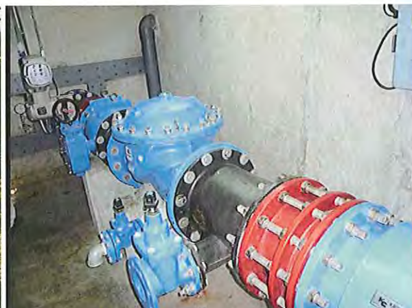
Remotely controlled water distribution valve
