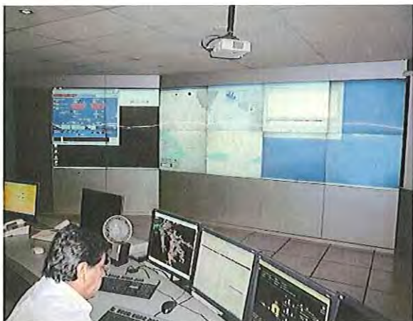
Remote control room at SEDAPAL's main office
