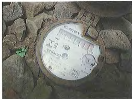
Water meter of SEDAPAL
