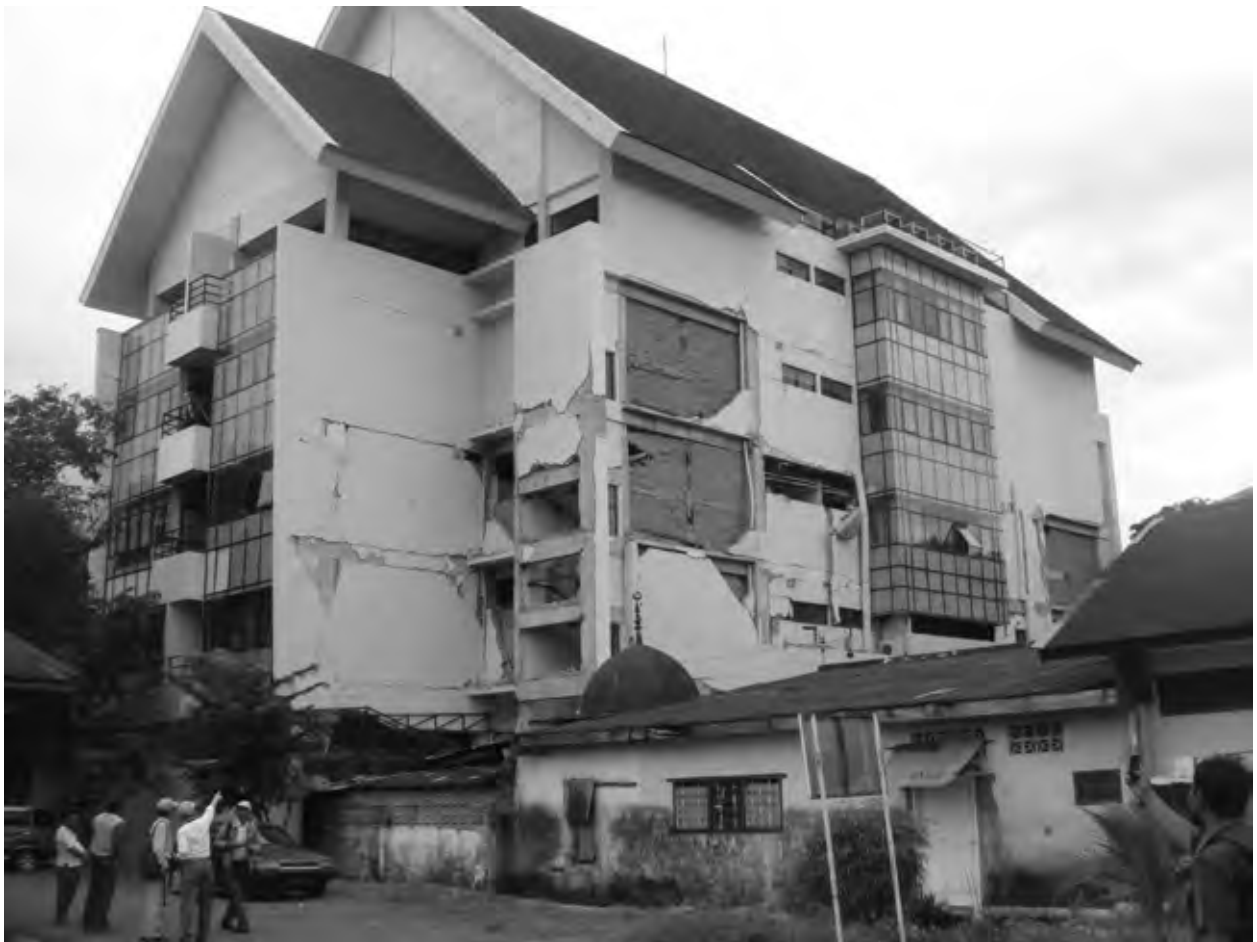
BPKP Building (Photo shows damage at the back side of the building)
