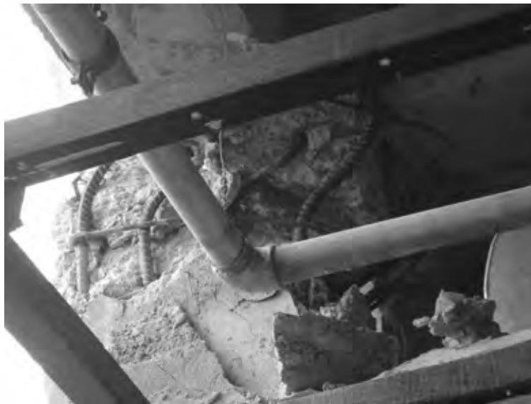
Photo of upper part column damage at Floor-2.
