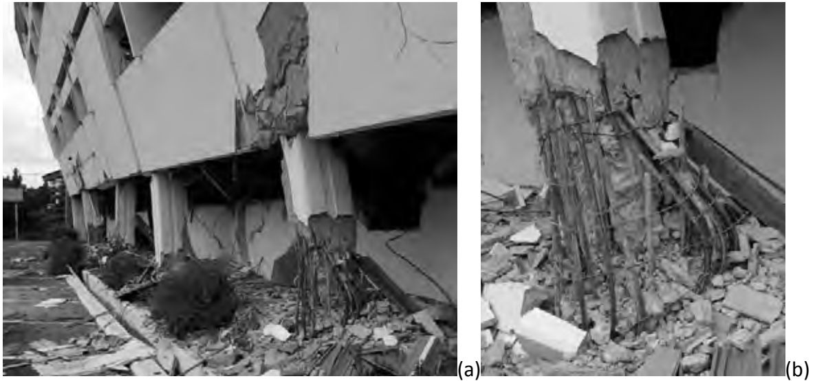
Damaged Columns (a) building side view (b) zoom view
