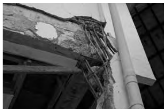
Figure 3.2.20 Deficient Re-bar Arrangement at the Column / Beam Joint
