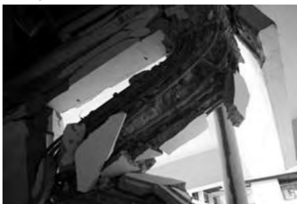
Figure 3.2.19 Inadequate Column Size and Inadequacy of Re-bars
