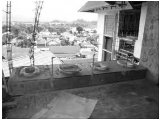
Figure 3.2.14 Collapsed Brick Wall of the rest room for females at the fifth floor
