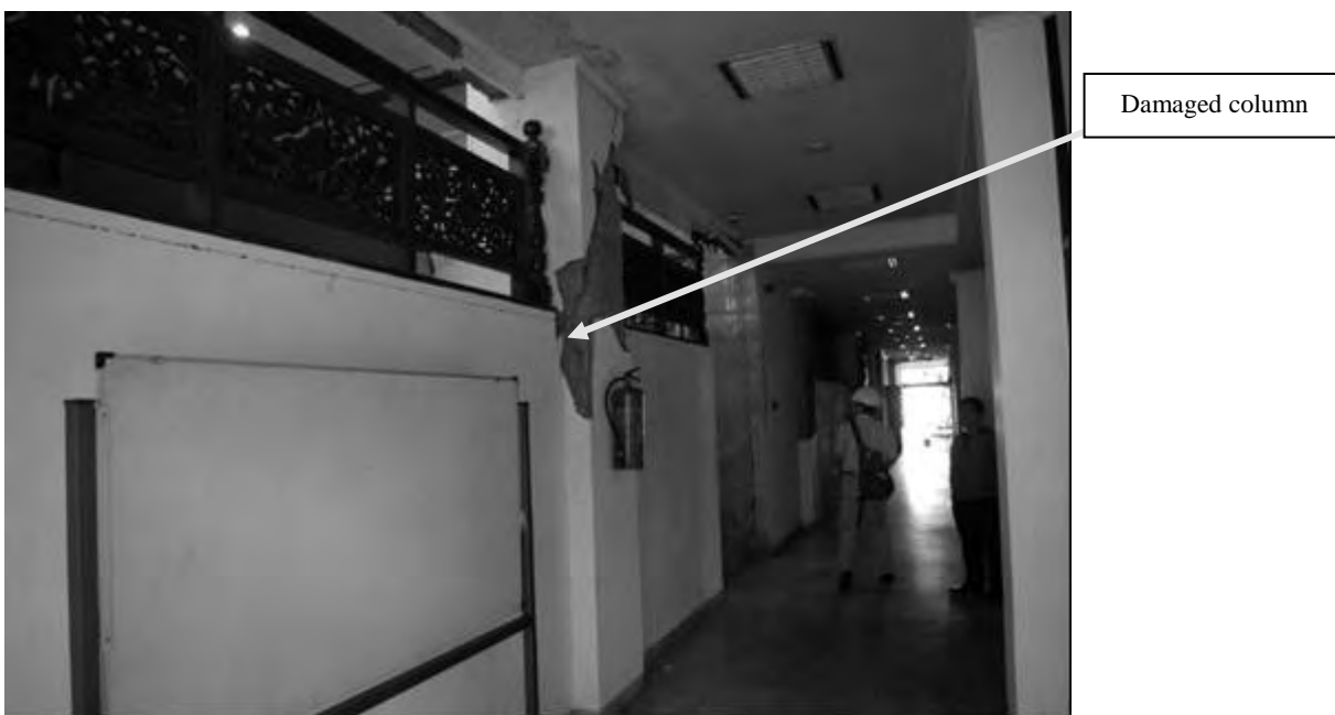
Figure 3.2.23 Level IV Damage to the Columns
