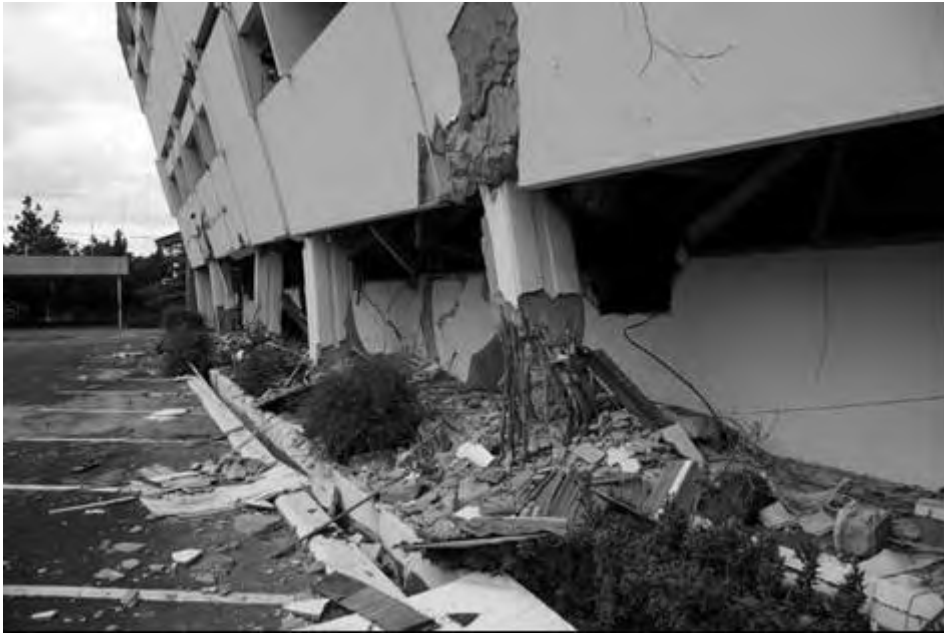
Figure 3.2.16 Photo Showing the Collapsed Brick Wall of the first floor
