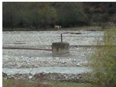
4. Connecting chamber of 7km site
