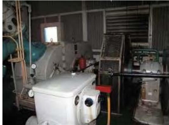
Figure D.18 Existing turbine and generator
