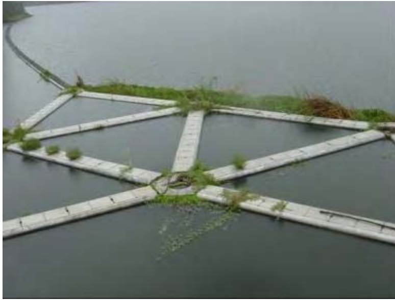
Figure 4.9 KGPS water intake screen (photo)
