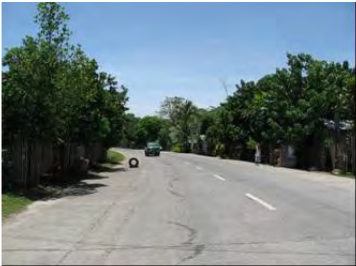
PHOTO.6.5.11-2 PORTLAND CEMENT CONCRETE PAVEMENT CONDITION
