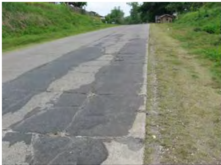
PHOTO.6.5.11-3 PORTLAND CEMENT CONCRETE PAVEMENT CONDITION
