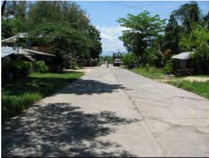
PHOTO.6.5.11-1 PORTLAND CEMENT CONCRETE PAVEMENT CONDITION
