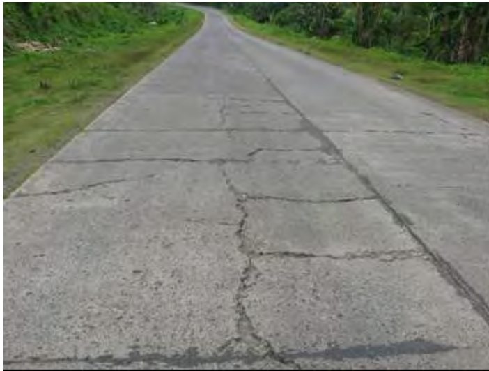
PHOTO.6.5.11-4 PORTLAND CEMENT CONCRETE PAVEMENT CONDITION
