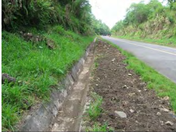
PHOTO.6.5.11-6 CEMENT CONCRETE DRAINAGE CONDITIONS
