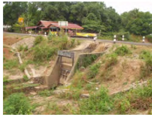
Flood gate without pump
