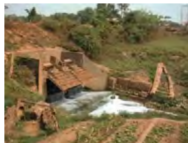
Flood Protection Gate in Savannakhet
