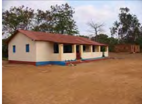
Health center after the repair. There is a nurses' accommodation next to the center.
