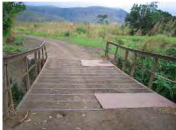
The repaired bridge. Circulation of farm products or people between Ndunguidi and Kimpese was improved
