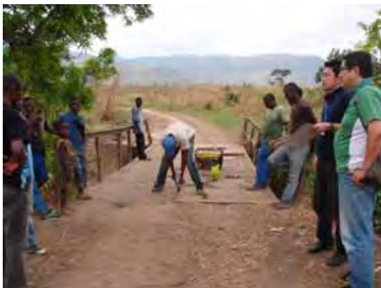
The bridge is repaired as a part of rehabilitation of feeder roads PP
