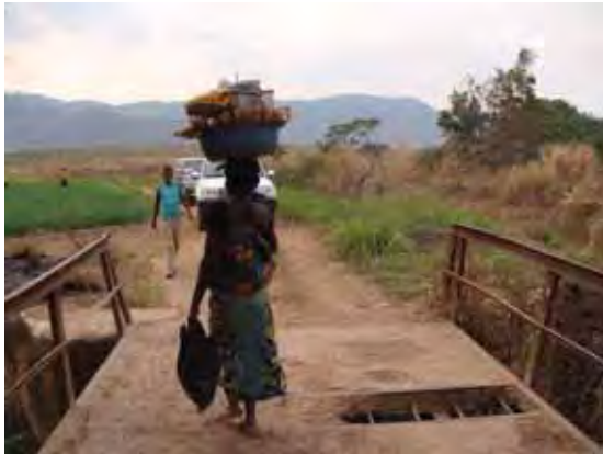
The bridge in danger to cross by the vehicle because of the holes
