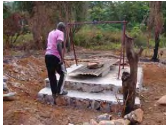
The well of Wene. The well of Wene. A well with pulley is easy to maintain.
