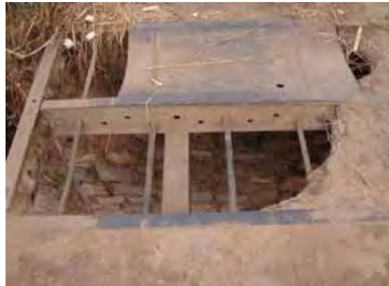
There were big holes before the repair
