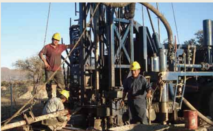
Using digging equipment provided by Japan to dig a well for people without access to safe water.
