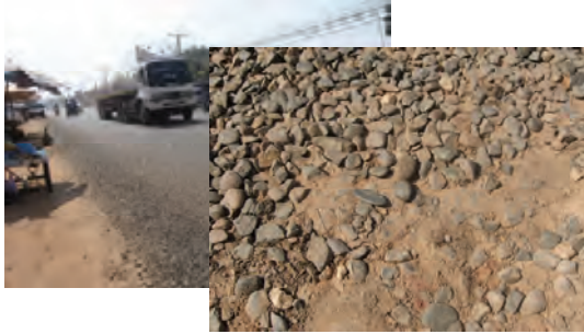
Deterioration of repaired pavement surface caused by the use of improper sub-grade material (Using uncrushed river gravel )
