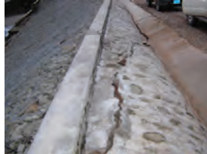
Damage (Crack) on Embankment due to improper compaction of fill material
