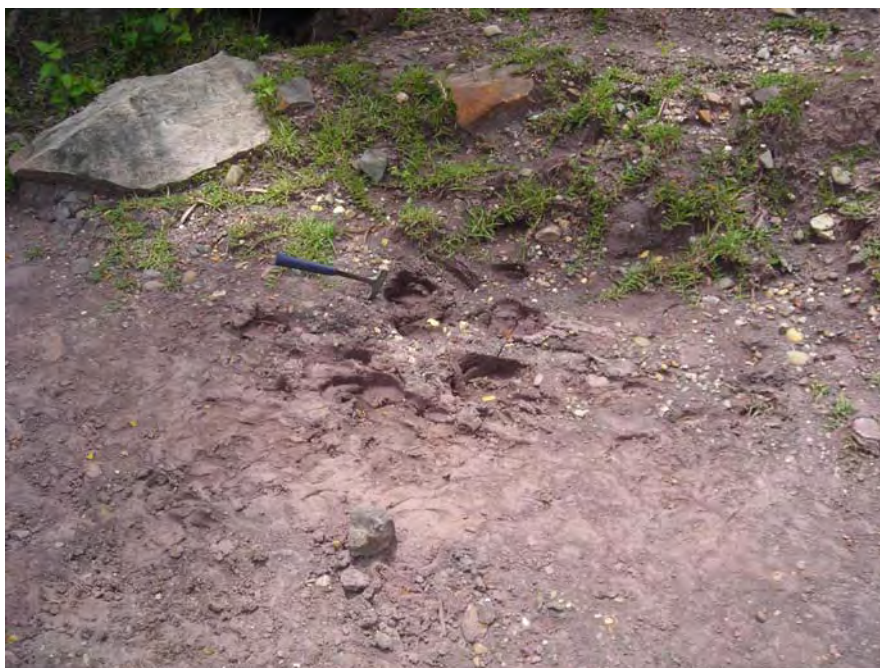
Mudstone foundation shows muddy condition wetted by rain.
