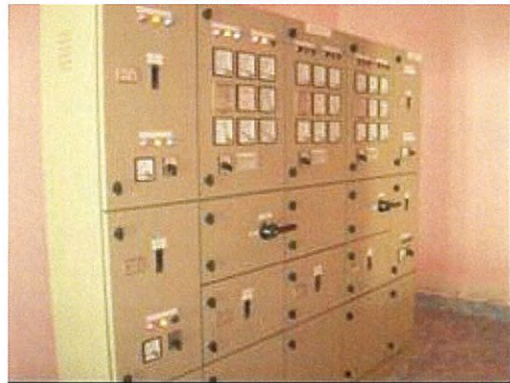
Generator Control and Distribution Panels
