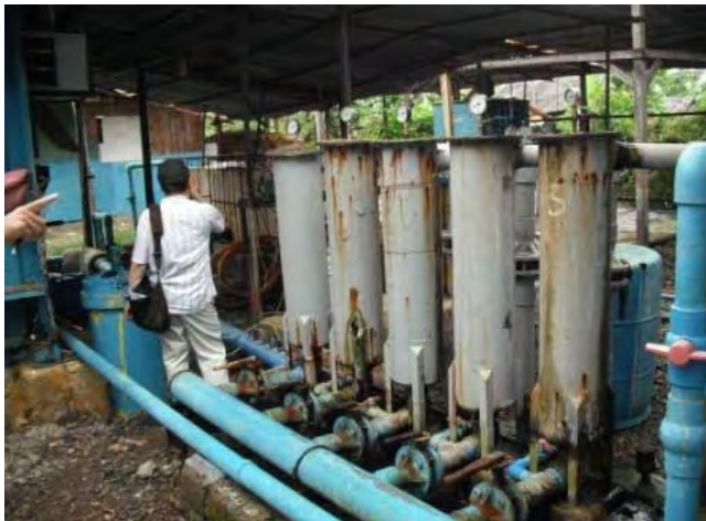
Desalination Plant of Mactan Rock Company (3)
