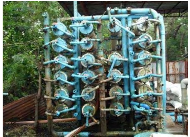
Desalination Plant of Mactan Rock Company (4)
