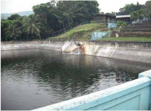
Tisa Water Treatment Plant (1)
