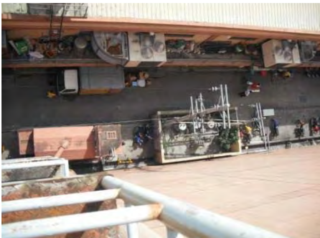
Electricity Receiving Facility Image
