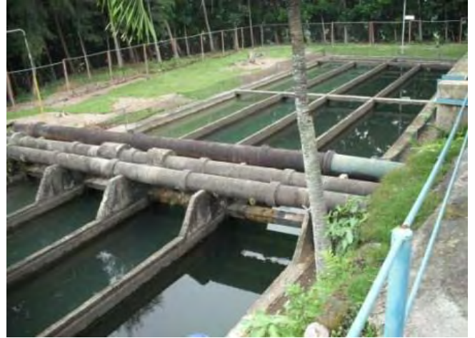
Tisa Water Treatment Plant (2)
