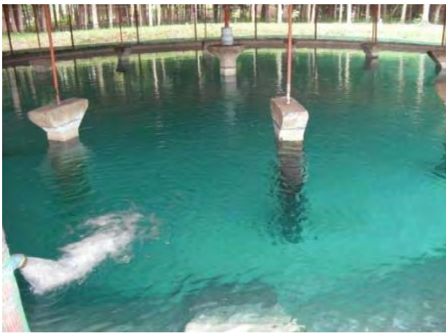
Tisa Water Treatment Plant (3)
