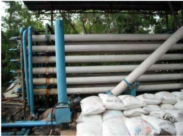
Desalination Plant of Mactan Rock Company (1)
