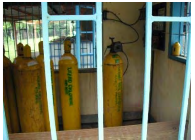
Tisa Water Treatment Plant (4)
