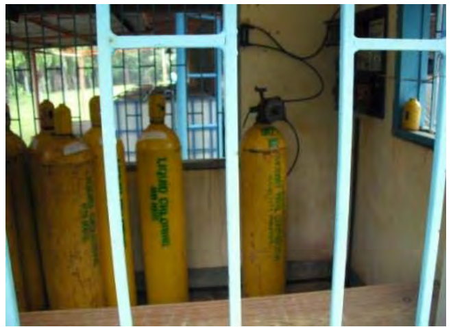
Tisa Water Treatment Plant (4)
