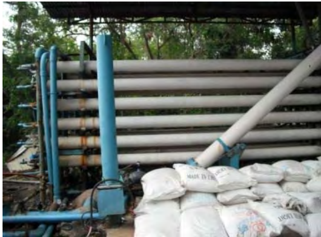
Desalination Plant of Mactan Rock Company (1)
