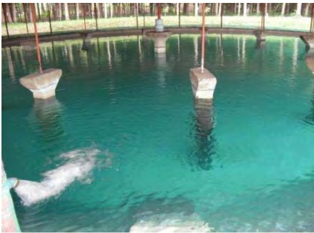
Tisa Water Treatment Plant (3)
