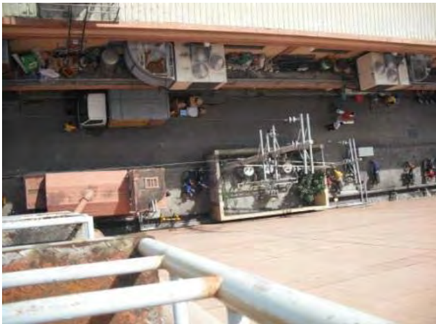
Electricity Receiving Facility Image
