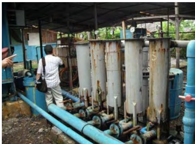
Desalination Plant of Mactan Rock Company (3)
