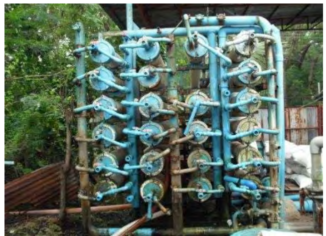
Desalination Plant of Mactan Rock Company (4)
