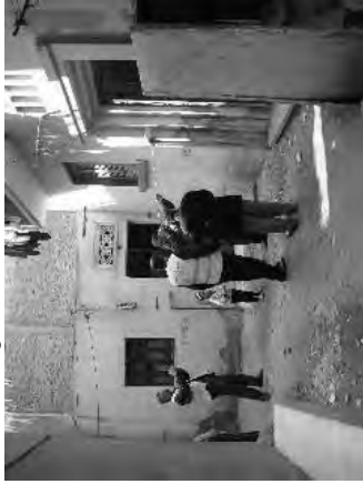
Figure 3-1 Detecting Leakage on House Connection by Acoustic Rod in Zagazig west A-3
