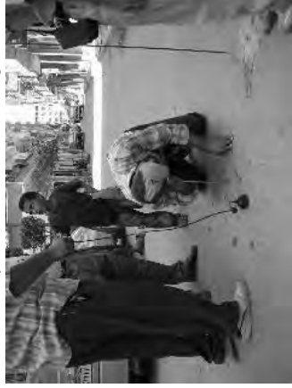
Figure 1-4 Method of Confirming Exact Location of Leak Point
