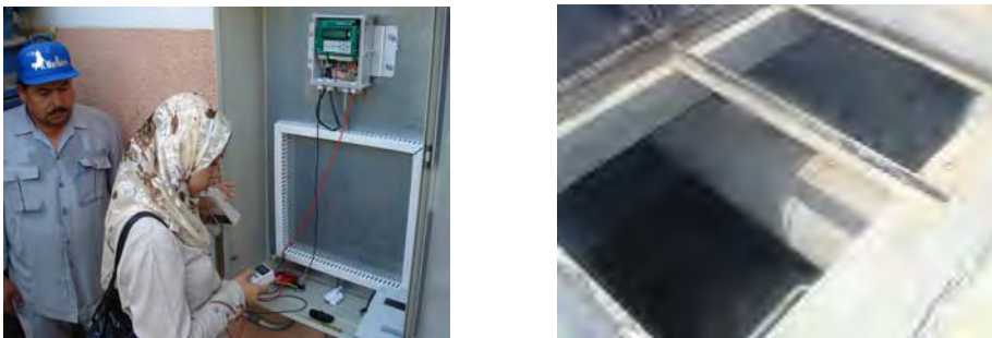
Figure 4.2-4 Installation Situation of Bulk Flow Meter in Abbasa WTP
