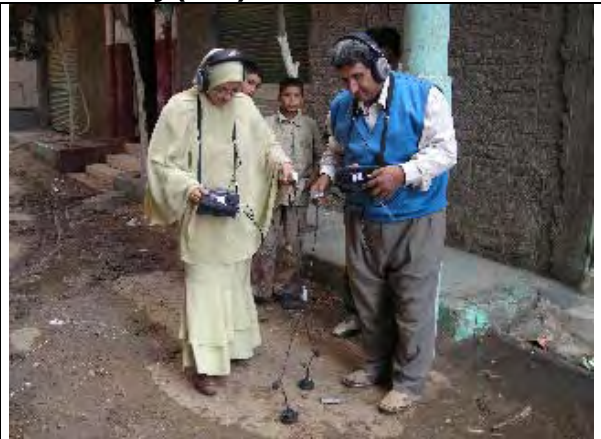
Counter part makes a search for the leak by water leak detector with Head of Hihya UFW team in Hihya Markaz. (Action U11). (Date: Nov. 26, 2007)
