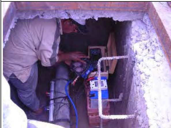
Installation of portable flow meter on MNF survey in Zagazig Markaz. (Action U2). (Date: Jun. 30, 2007)
