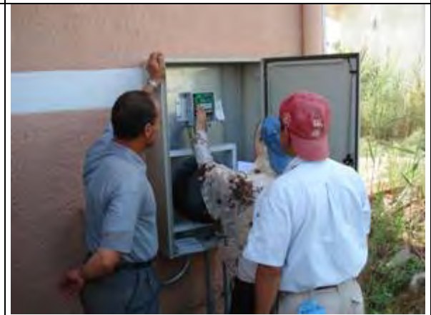
Training of installation of data roger, data reading and data transportation in Abbssa W.T.P (Action S3.5). (Date: July.14, 2008)
