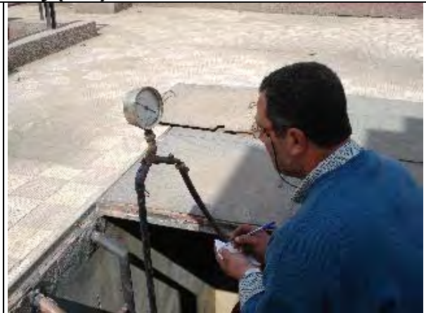
Counter part measures and records the water pressure in Zagazig W.T.P. (Action S2.6) (Date: Feb.20, 2007)
