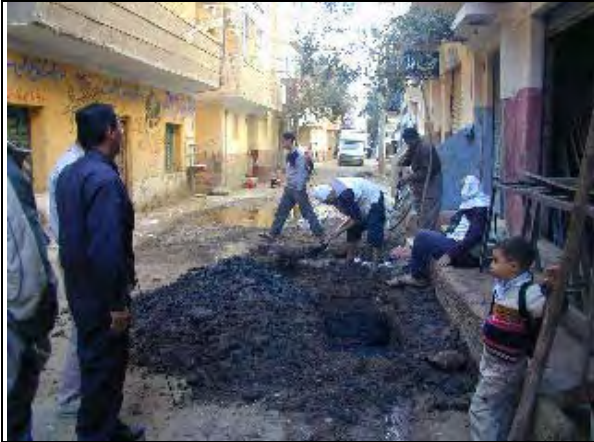
Excavation of leakage point found by counterpart team in Hyhya Markaz. (Action U12) (Date: Dec. 13, 2007)
