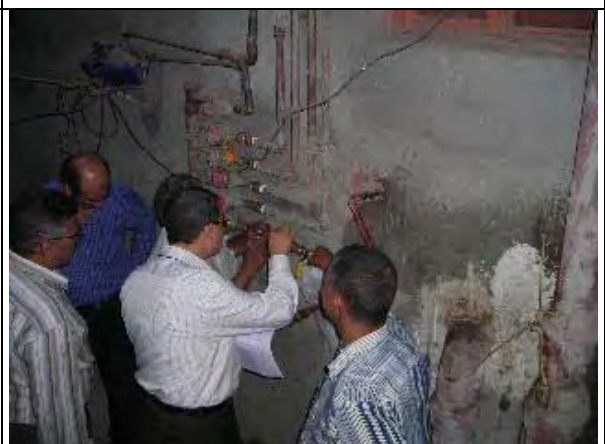
Investigation of meter error in Zagazig City East. (Action U7&8). (Date: Nov. 10, 2007)
