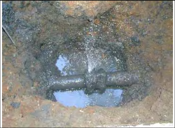
Leakage point found by counterpart team in Hyhya Markaz. (Action U12). (Date: Dec. 13, 2007)
