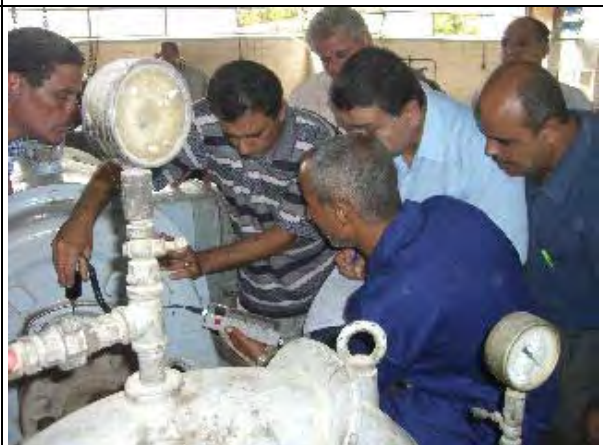
Counter parts record the vibration of motor at before maintenance and after maintenance in Abbasa W.T.P. (Action S2.4.6) (Date: Sep.5, 2007)
