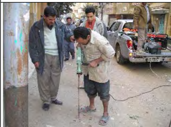
Counter part makes a hole at suspected leakage point by drill hummer in Hihya Markaz. (Action U11). (Date: Dec. 8, 2007)
