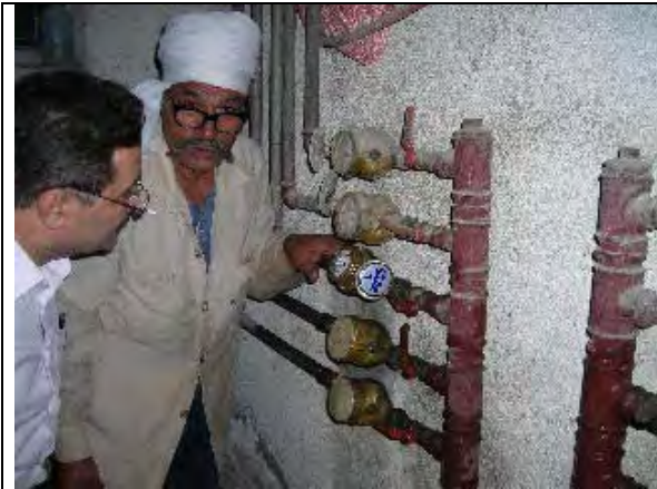
SHAPWASCO replace to new water meter in Zagazig City East. (Action U7&8). (Date: Nov. 12, 2007)
