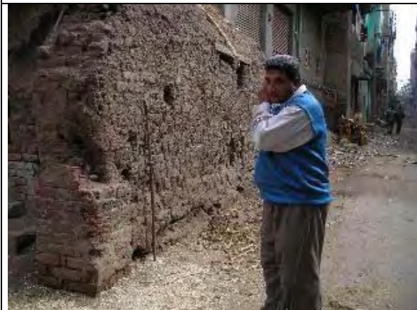
Counter part makes a search for the leak by acoustic rod in Hihya Markaz. (Action U11) (Date: Nov. 29, 2007)
