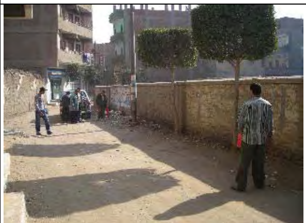
Counter parts investigate the pipe and cable under the ground by locator in Hihya Markaz. (Action U11). (Date: Dec. 13, 2007)
