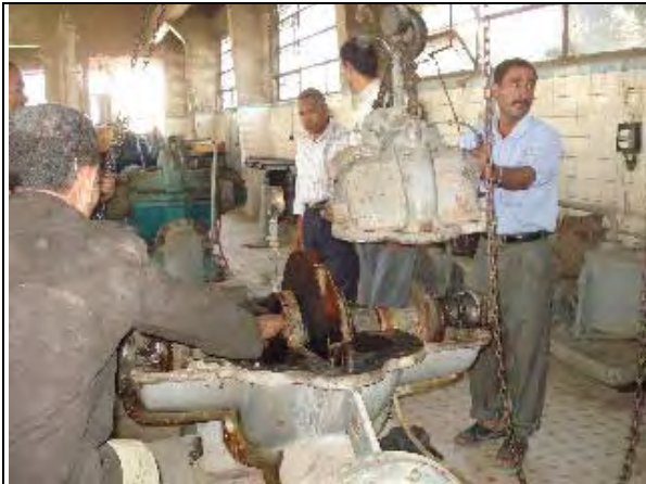
Counter parts apply a SOP to pump maintenance in Abbasa W.T.P. (Action S4.6) (Date: Sep.5, 2007)
