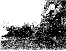
1) Water visible leakage at Zagazig City Time : 10:30 AM (12:50 received call) at 11:15 AM Address : 3rd street - mohamada District in front of fire fighting station Excavation for repair finished around 12:00
