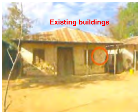
“X” mark on the building wall
