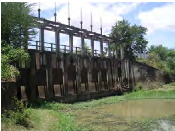
Existing Ream Kon Headworks (Ream Kon Sub-project)
