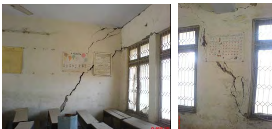
Fig. 6-4 Photo of Damaged Structure in Govt. Girls High School
