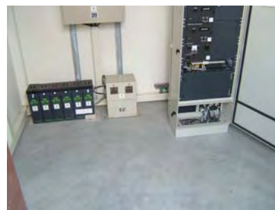
Warning Post (after)
