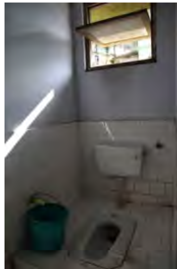
Broken flush lever (no water)
