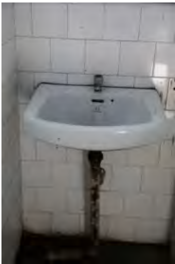
Broken sink without water
