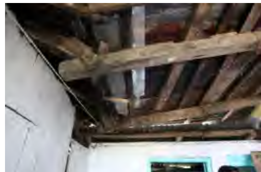
Block Officer's residence with broken roof
