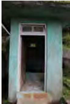
Unmaintained public convenience
