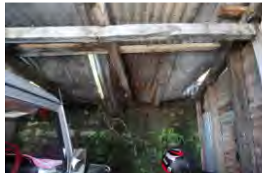
Broken tin roof of garage
