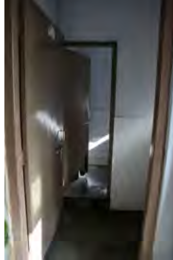
Decayed toilet doors
