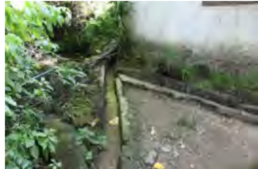
Forest guard's residence without proper drainage
