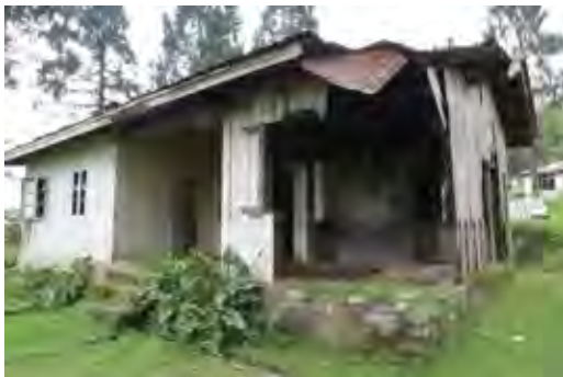
Office abandoned after fire
