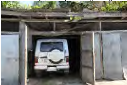
Old garage with broken tin roof
