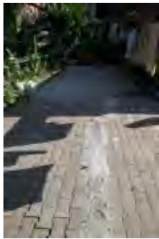
Landslide at Forest Guard's residence
