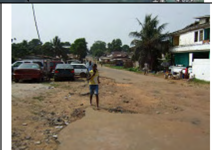
Inundated place, due to insufficient flow capacity of drainage near 18 th Street
