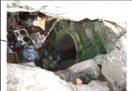
Many garbage are thrown around broken underground pipe for drainage.
