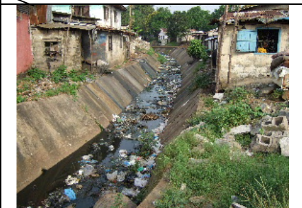
Main channel of Soniwein with concrete lining covers concrete roof in downstream
