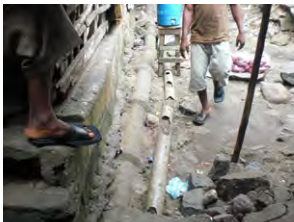
Figure 2.5-9 Damaged PVC Pipelines (Right)
