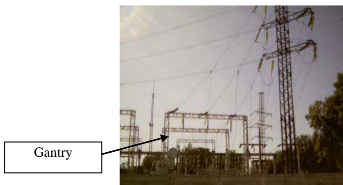
Figure 1-3-1 Connection point between the existing transmission line and switchyard
