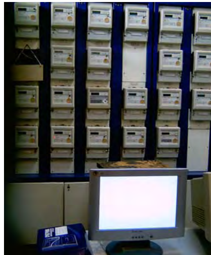
Figure 2-1-6 Data monitoring system
