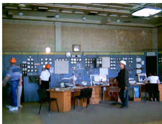
Figure 2-1-3 Central operation room
