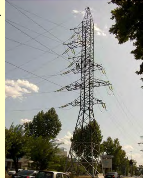
Standard T-junction tower
