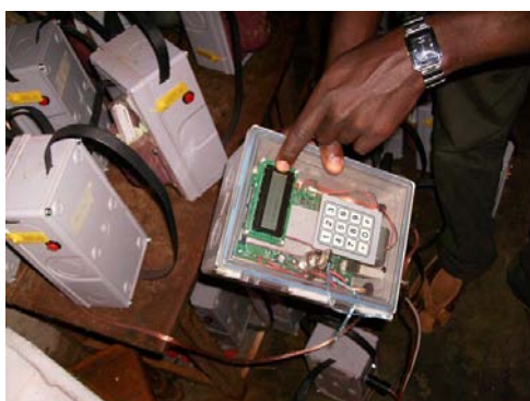
Charging Control made with Registered No. of Lanterns
