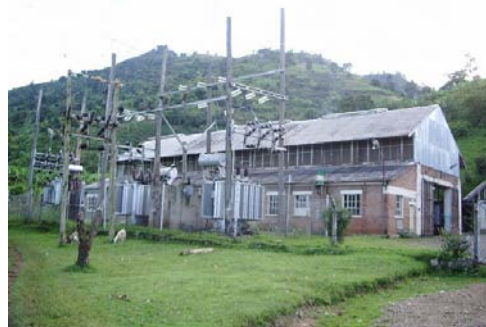
Power 5.4 MW (3 Unites x 1.8 MW)
