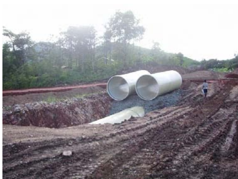
Pressure Pipe Line (Discharge 10m 3 /sec, Head 160 m)
