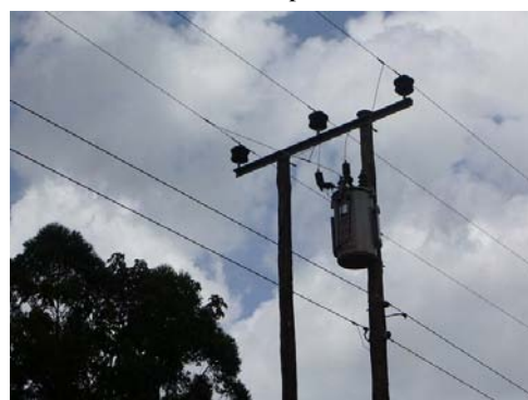
33 kV Transmission and 240 V Distribution Lines
