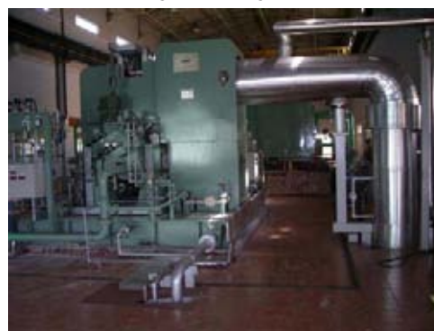
Steam Turbine and Generator of 16 MW
