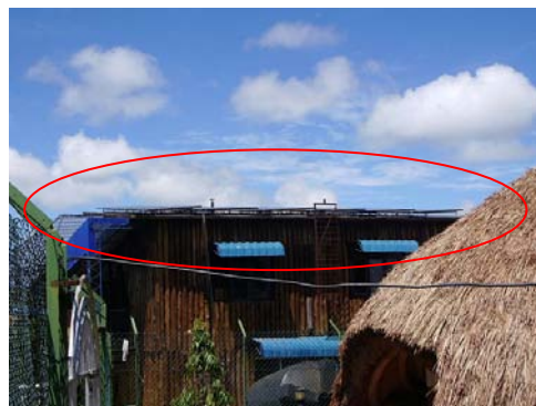
Hotel with 20 Sets of PV Modules of 80/85 W
