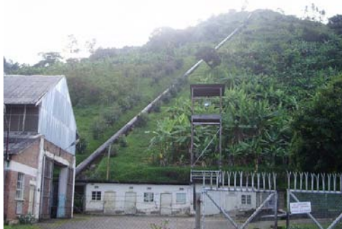
Steel Pipeline and Power Station (Kilembe Mines Ltd.)
