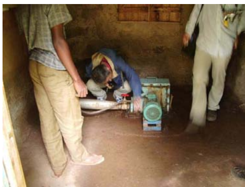
Turbine/Generator of 1.5 kW operated for 2 hours each Morning and Evening
