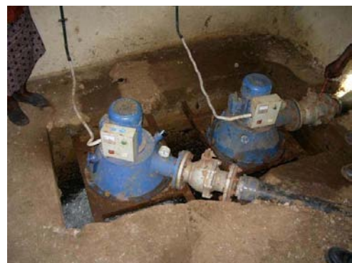
Turbines/Generators mad in China (1 kW x 2 Nos.)
