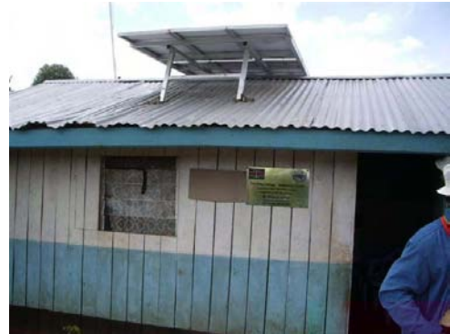
PV Modules (500 Wp)
