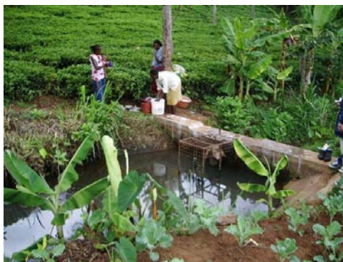
Intake Weir in a Stream of 2 m Wide
