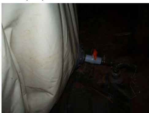
Tank for Gas Produced (4m 3 )
