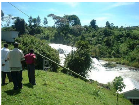
Steel Pipe Lines and Powerhouse
