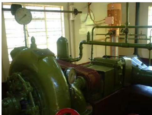
Hydraulic Turbine and Generator
