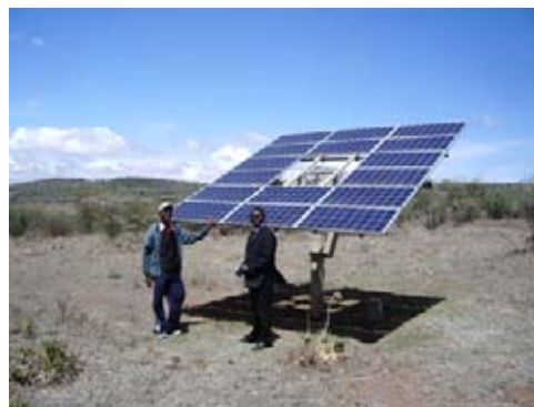
PV Modules for Lighting in Lodge (1,280W)
