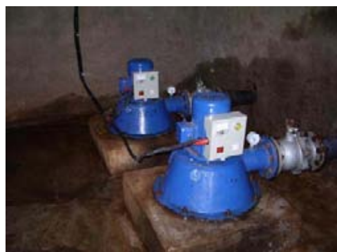
Turbines/Generators made in China (1 kW x 2 Sets)
