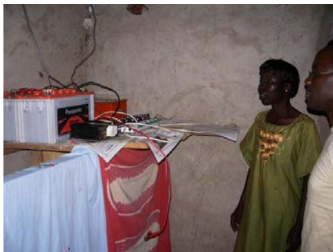
Charging Facility of Kochia Development Group
