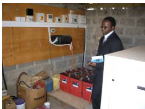
Batteries (12 nos. x 350 Ah) and Standby Generator (12.5 kVA)
