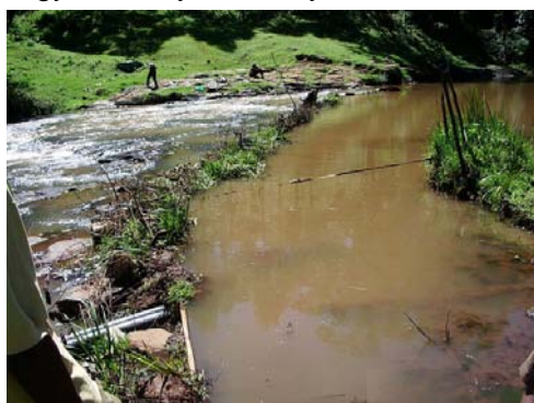
Intake and Waterway of PVC Pipes in Chemosit River
