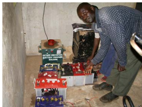
Monthly Electricity Fee at Ksh 500, Charging Business Income at Ksh 6,000
