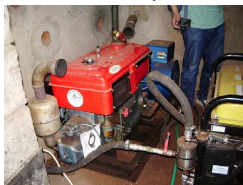
Methane Gas Generators (10 kW x 2 Sets)
