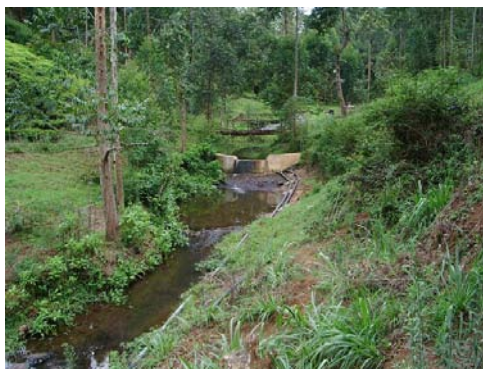
Intake and Pipelines (PVC 150 mm) of Small Hydro
