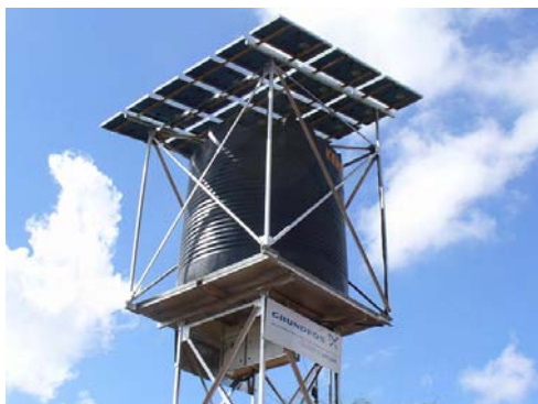
PV Modules and Water Tank
